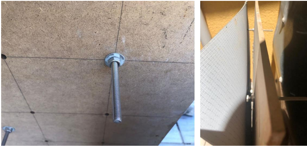
Figure 20: Pin system details. Bolt, nut, and washer combination on the support surface.
