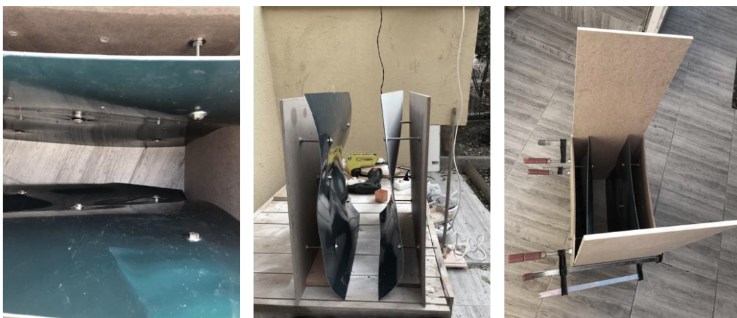
Figure 21: Details and arrangements for concrete production with the formwork, developed and photographed by the author.
