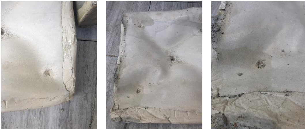
Figure 36: Horizontal plastic seal material details on the concrete surface produced and photographed by the author
